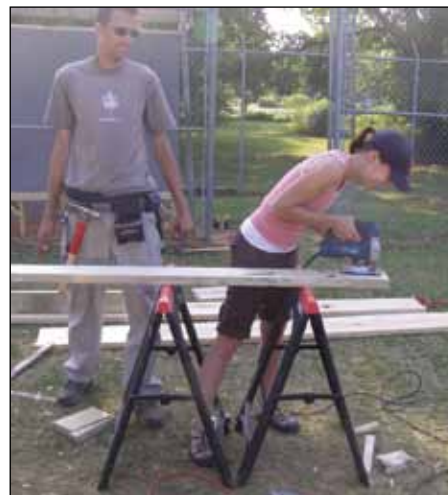
Chad Vickery (left) jokes with Leah Teuber as she cuts rafters for the rebuilt dugouts in Hale County.
