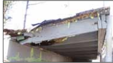
What the home dugout roof looked like at the Curtis Smith Baseball Field in Greensboro before the student engineers went to work in March 2007.
